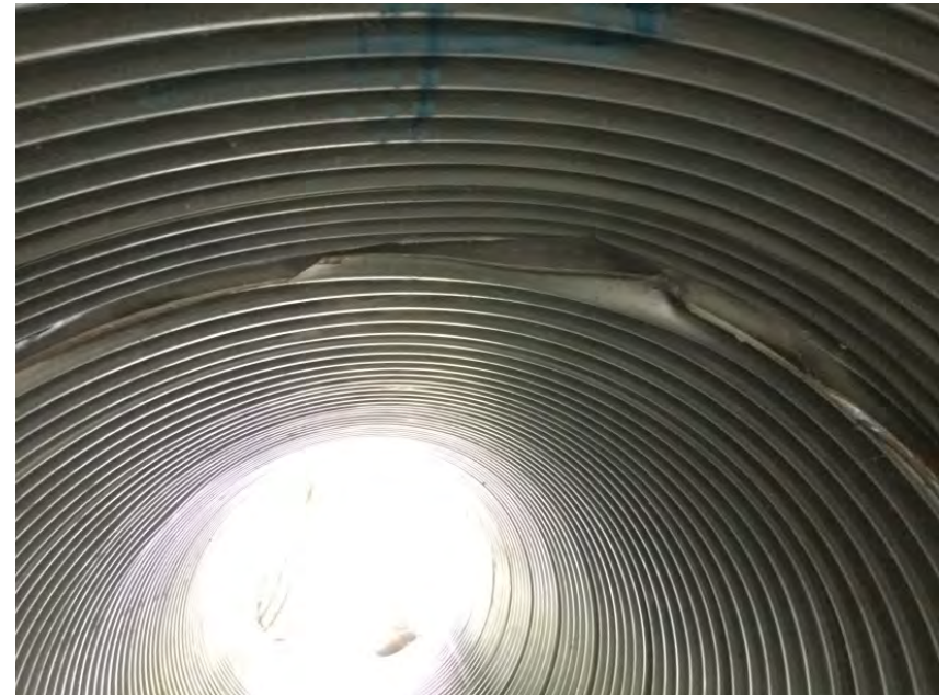
Damage at coupler location
